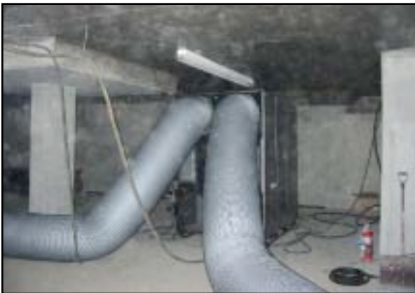
Underground 45,000 SQ. FT. (1 heater)
